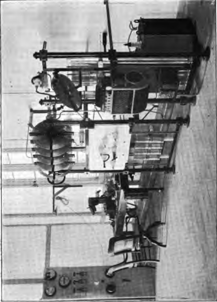
FIG. 140.—2.5 T.K. station at Ambon (Dutch East Indies).
